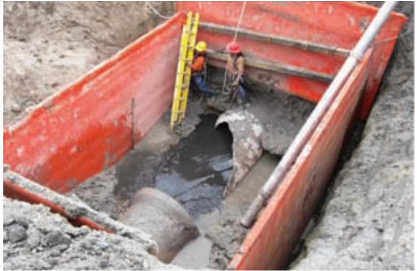
Failure of 1,215mm RC main sewer
